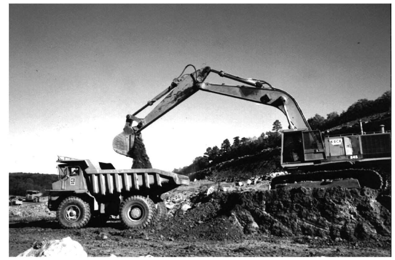
State Highway 82 construction. View to the N.E., SW 1/4, SW 1/4, sec. 8, T. 7 N., R. 21 E., Haskell County, Oklahoma, 10-12-94.
