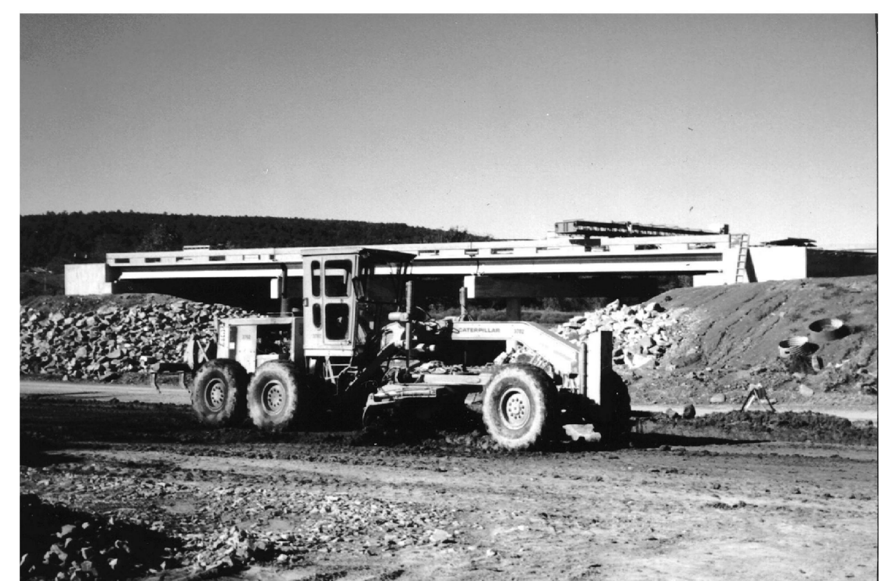
State Highway 82 construction. New bridge over Andrew Creek, SW 1/4, SW 1/4, NW 1/4, sec. 8, T. 7 N., R. 21 E., Haskell County, Oklahoma, 10-12-94.
