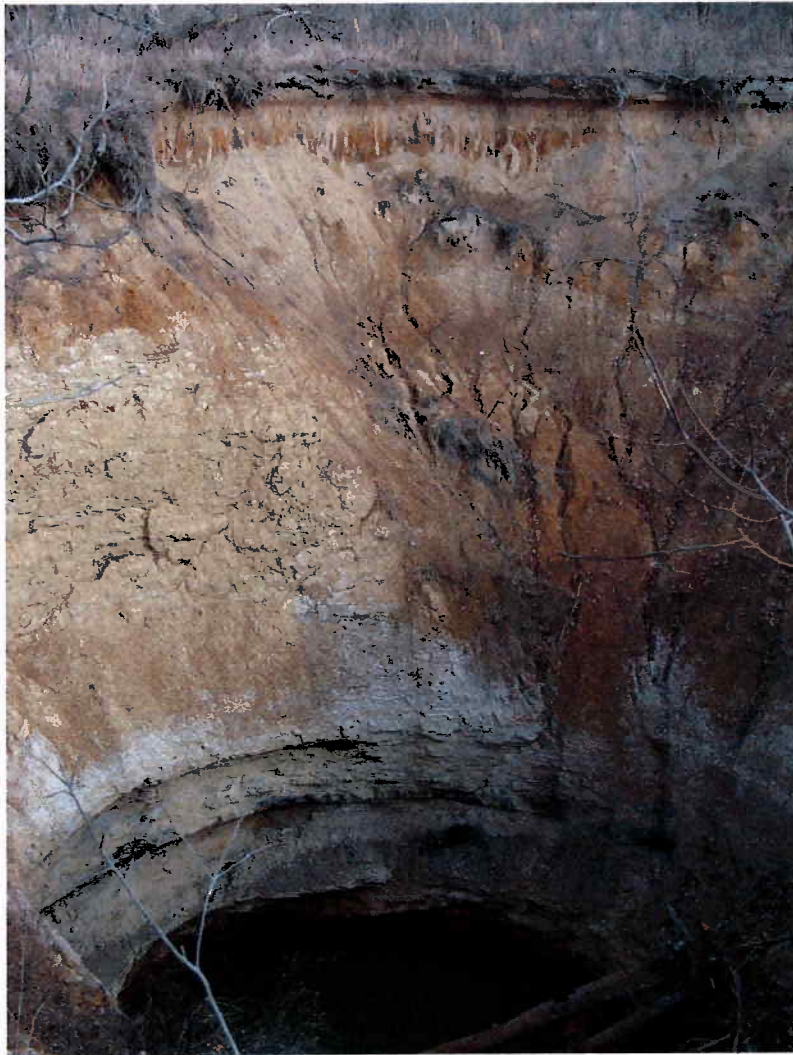
Fig. 3. Large shaft collapse on the Harrisburg lease (T29N, R23E, sec. 19, no. 43).
